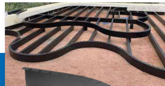
Curved Rim Joist
